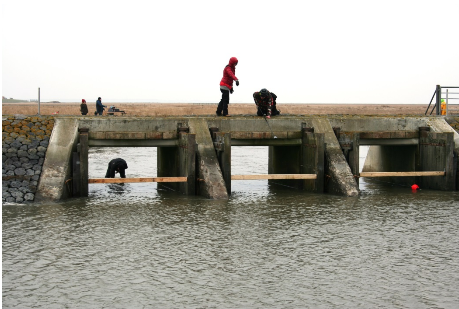
Figure 5-3: Open gates at the tidal channel system “Osterwehl” (Langeness). Gates are fixed by wooden beams against a closing by water inflow. Photo by M. Deicke (2013).
